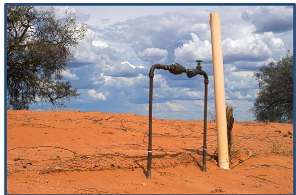
A water pipe, a tap and a meter
